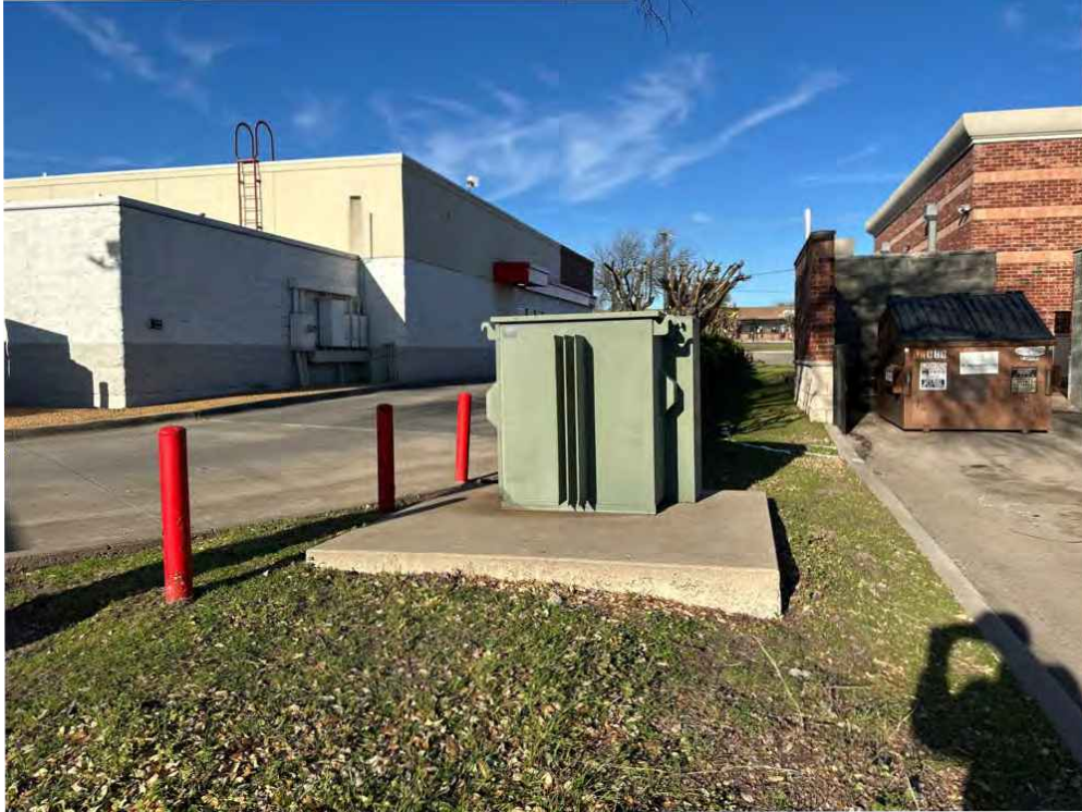
Photo 9 - View of the pad-mounted electrical transformer to the southeast of the building.
